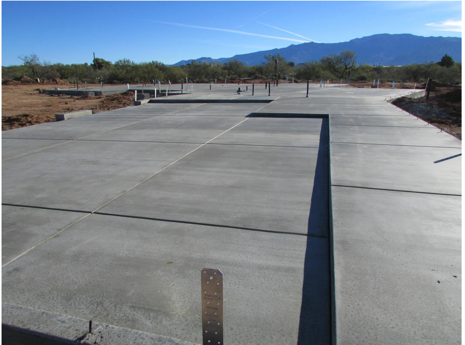
Engineering from the dirt below to the trusses above. You can see a “shear wall” hold down in the foreground.
